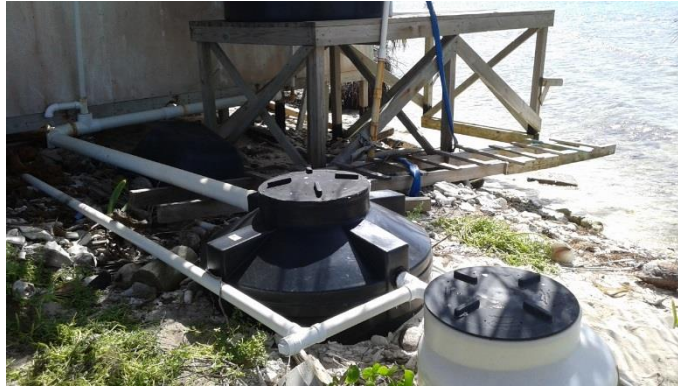
Figure A-1: Semi-Anaerobic Biodigester (Black) and Upflow Rock Clarifier (White) at Laughing Bird Caye (Photo taken by Christine Prouty)
