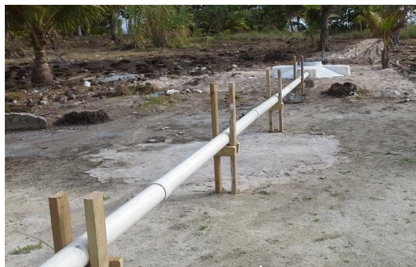
Figure A-7: Distribution System from Ranger Facility to WWTS at Little Water Caye (Photo taken by Christine Prouty)
