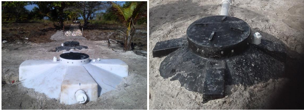
Figure A-5: Semi-Anaerobic Biodigesters in Series at Little Water Caye (Photos taken by Christine Prouty)
