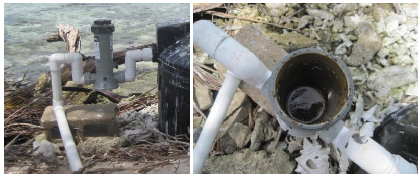
Figure A-11: Chlorine Contact Chamber (Without Tablets) at Silk Caye (Photos taken by Christine Prouty)
