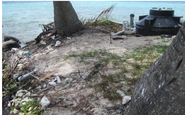
Figure A-8: Wastewater Treatment System at Silk Caye (Photo taken by Christine Prouty)
