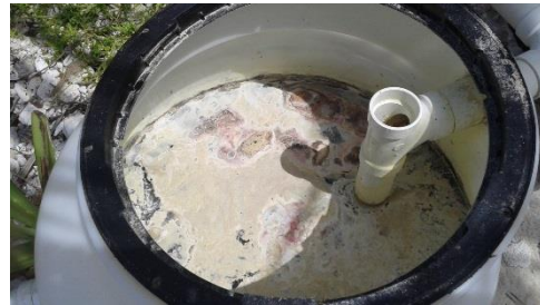
Figure A-3: Inside of Upflow Rock Clarifier at Laughing Bird Caye (Photo taken by Christine Prouty)
