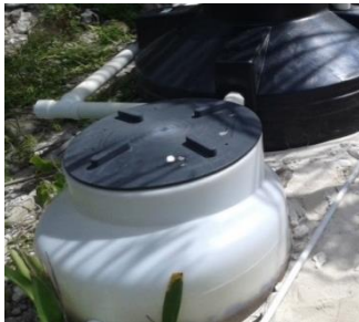
Figure A-2: Upflow Rock Clarifier at Laughing Bird Caye (Photo taken by Christine Prouty)
